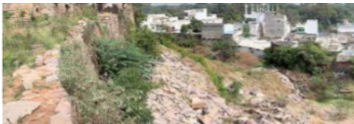
Under siege: A view of the damaged portion of the moat wall at the Golconda Fort in Hyderabad. •SPECIAL ARRANGEMENT
